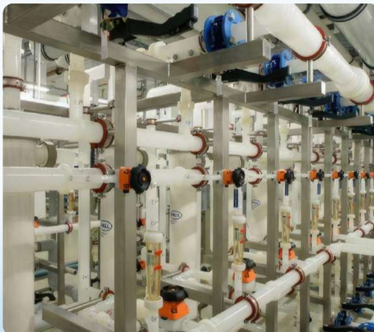
UPW production plant
